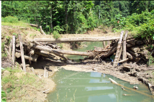
Plate 3 Old river crossing not decommissioned.
