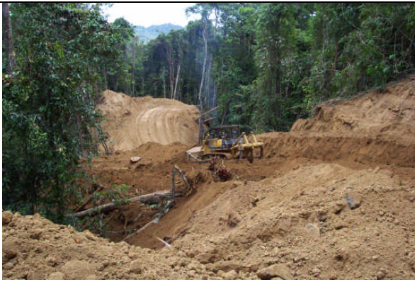
Plate 1 Road construction in contravention of court order.
