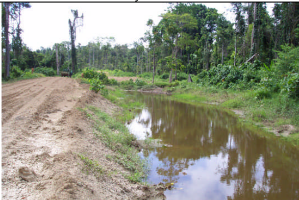
Plate 3 Lack of proper drainage causing ponding.
